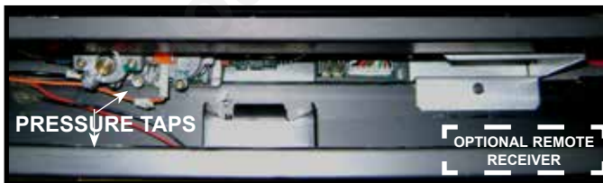
Figure 11.5 Valve Pressure Taps and Remote Receiver Location
