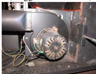
(Plugged Exhaust Fan)
