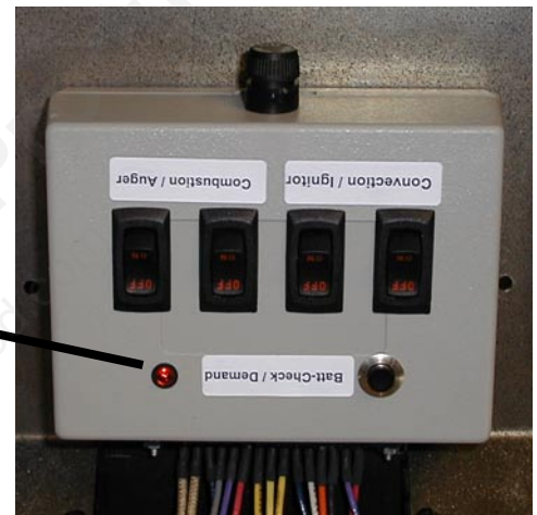
TEST BOX (AS IT IS INSTALLED IN THE STOVE)
