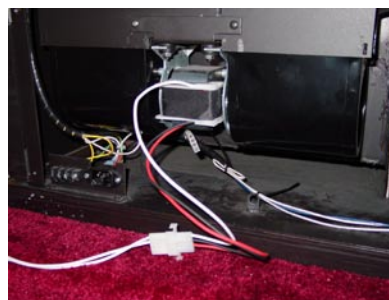
TEST CORD CONNECTED TO THE BLOWER
