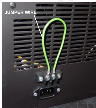
THERMOSTAT BLOCK WITH A JUMPER WIRE ATTACHED.
