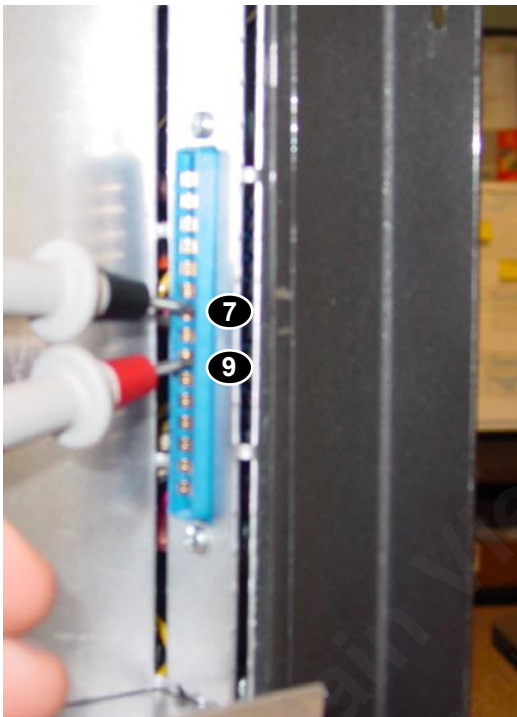
TESTING FOR CONTINUITY ON PIN 7 & PIN 9 IN THE JUNCTION BOX.
