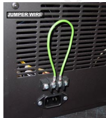
THERMOSTAT BLOCK WITH A JUMPER WIRE ATTACHED.
