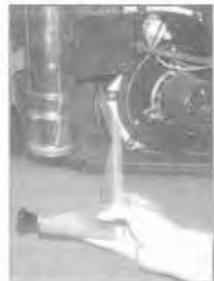
PHOTO A (damper position behind firebox)
