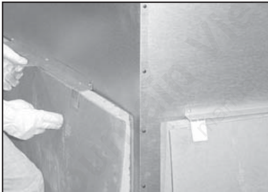
Figure 4.5 Unpacking Back Refractory
