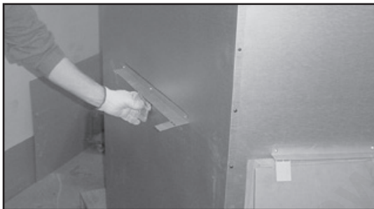
Figure 3.7 Bend Refractory Brackets Back Down
