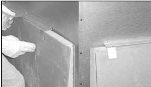
Figure 3.5 Unpack Back Refractory
